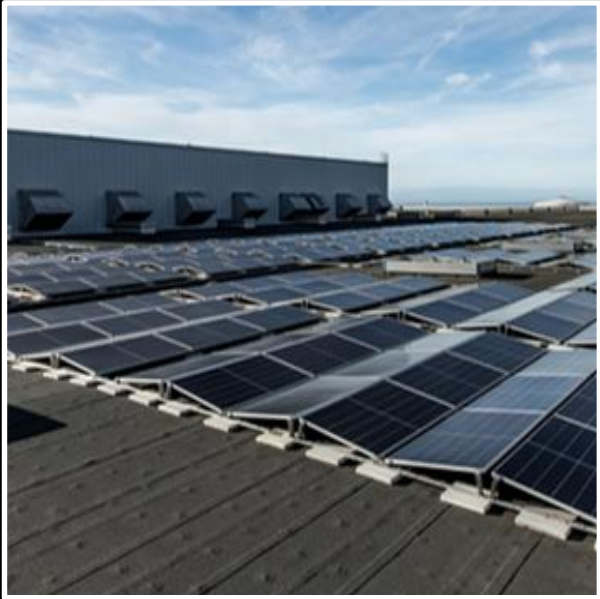
PV extension by 2MW
